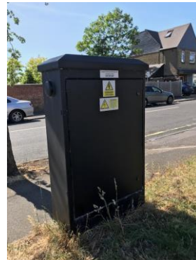
Typical Feeder Pillar
