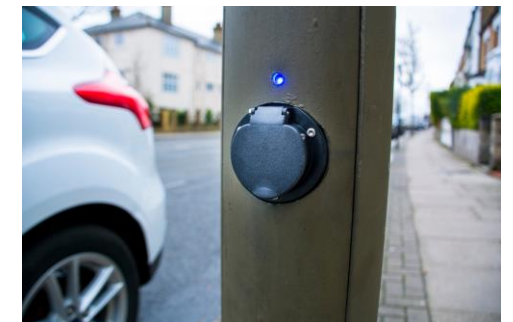
An example of a retro fit to an existing street light
