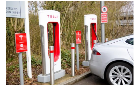
An example of multiple EV rapid chargers
