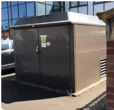
Typical GRP substation for UK Power Networks and customer
