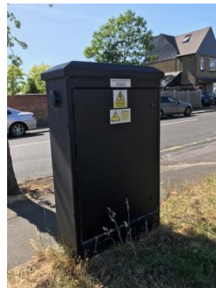
Typical Feeder Pillar
