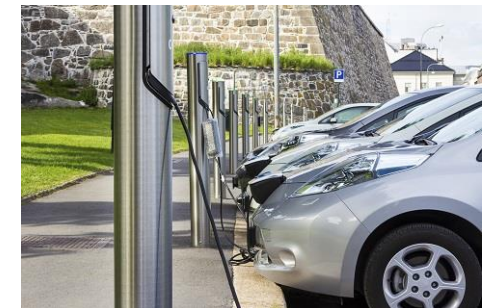
An example of EV chargers installed in a car park
