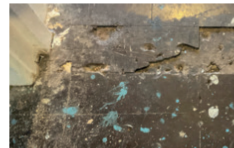
Asbestos containing floor tiles and bitumen adhesive
