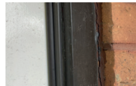
Asbestos containing mastic to window frame
