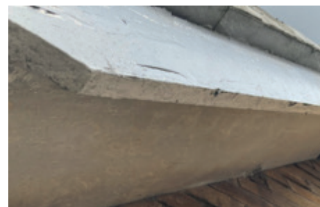
Asbestos cement soffit board to roof
