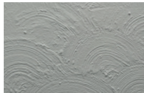
Asbestos containing textured coating to ceiling (ARTEX)
