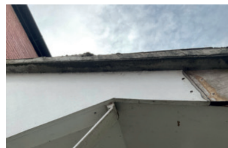
Asbestos containing cement undercloak to canopy
