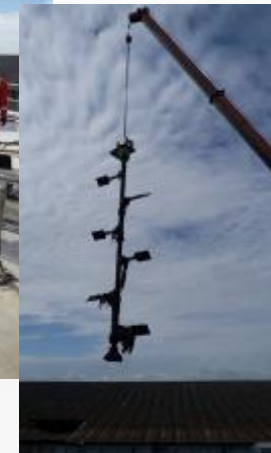
Future biogas changing feed critical Digester Stirrer when bottom bearing showed signs of failure. The digester was off line for 12hrs . Parts in stock and engineers on site next day with a crane.
