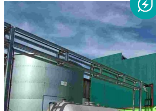
Biomass Boiler at Bel Plant Tangier, Morocco
