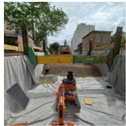
Figure 5: Excavation of a trench prior to its backfilling with porous materials and construction of the trackform
